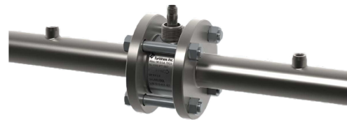
Installed SLGM0200L Slim Line Meter
